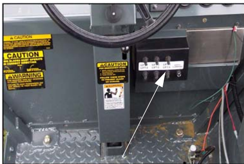
Depth Command Switches (Located near the operator's station) -Typical View
