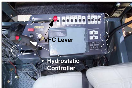
Circuit Breakers (Located on side console) -Typical View
