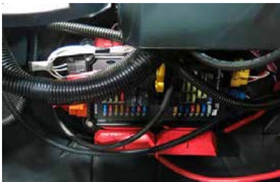
Fuse/Relay Box (Cover Removed) -Typical View
