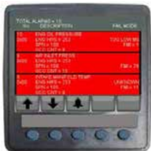
Active Alarm Screen -Typical View
