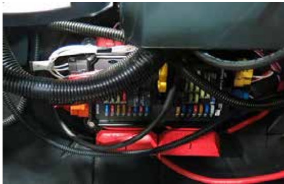
Fuse/Relay Box (Cover Removed) -Typical View
