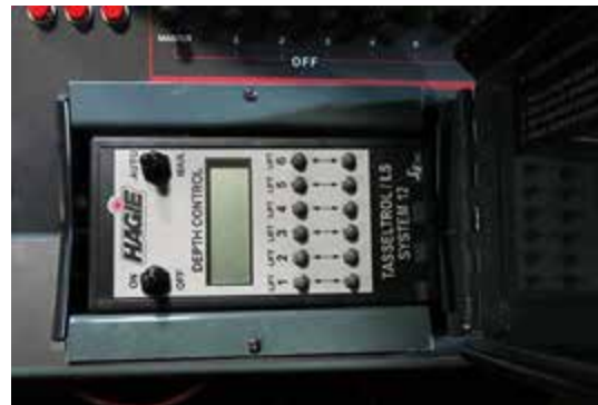
Tasselrol/LS System 12 Control Panel (Located on the side console - lift cover to access) -Typical View
