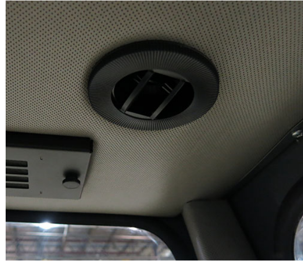
Air Vent -Typical View
