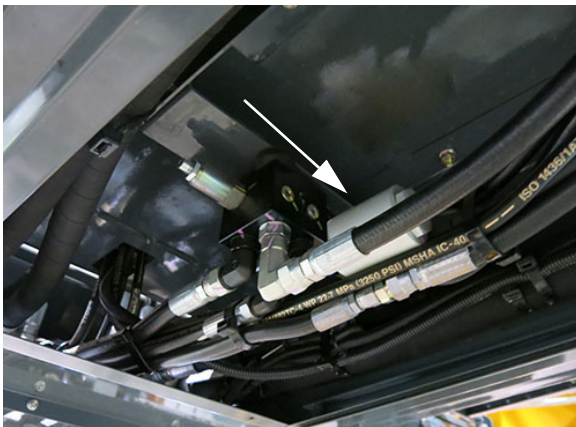
High Pressure In-Line Filter (Located beneath machine - lower front screen panel out to access) -Typical View
