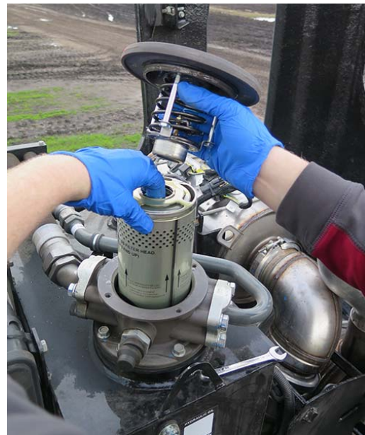
Return Filter 1 (Located inside filter housing on top of hydraulic oil reservoir - open hood to access) -Typical View
