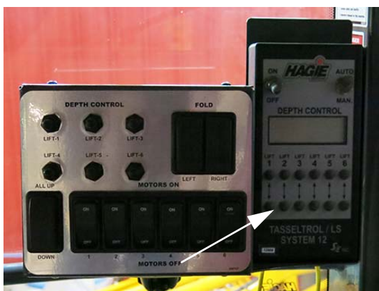
Tasselrol/LS System 12 Control Panel -Typical View
