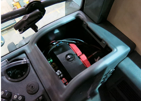
Circuit Breakers/Fuses (Interior) (Located rear of side console - remove tray to access) -Typical View
