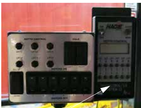
Tasselrol Control Panel -Typical View
