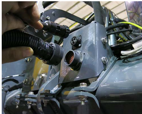
Electrical Connections (Right-hand side of machine shown) -Typical View
