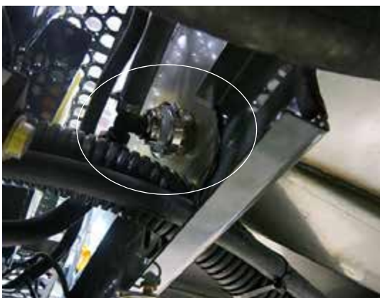
Jet Agitator (Located on each end of the solution tank) -Typical View
