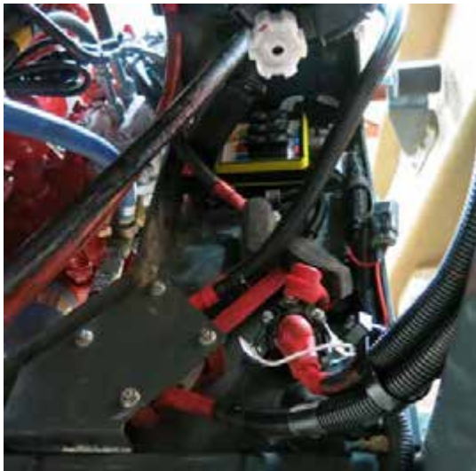
Tier 4 Final Engine Fuse/Relay Block (Located beneath batteries on the rear left-hand side of machine) -Typical View * View shown from beneath machine
