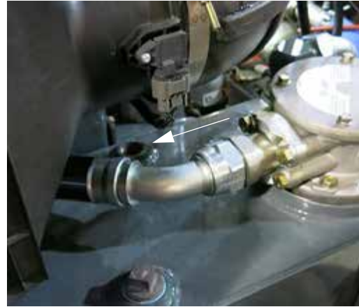
Breather Cap Removed -Typical View
