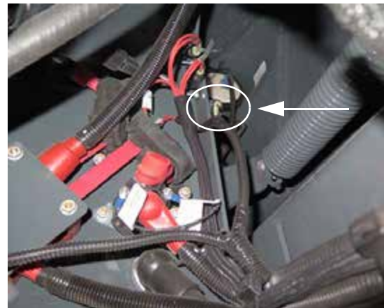
Hood Actuator Fuse (Located beneath rear left-hand side of machine) -Typical View
