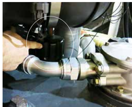
Breather Cap (Located on left-hand side of machine near return filter housing) -Typical View
