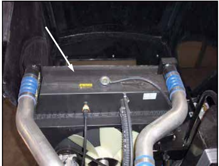
On engine compartment, near radiator cap.
