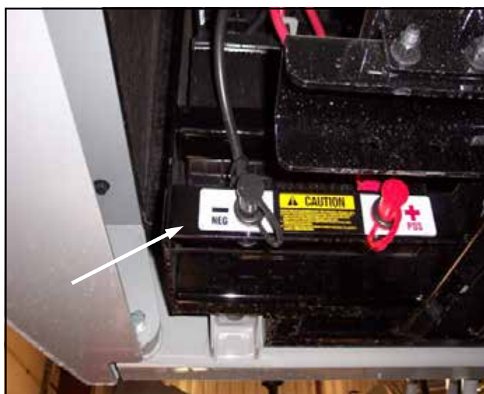
Rear of mainframe above booster terminals.
