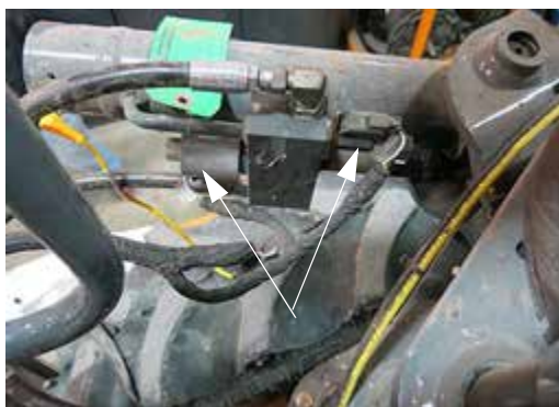
Lock Valves -Typical View
