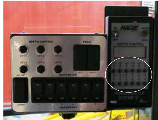
Lift Up/Down Switches (Located on the Tasselrol Control Panel) -Typical View
