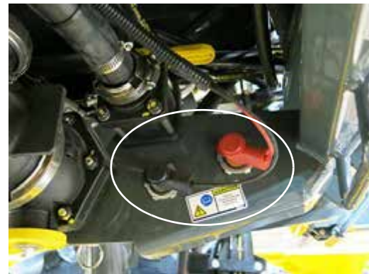
Power Ports (Located near front fill assembly) -Typical View
