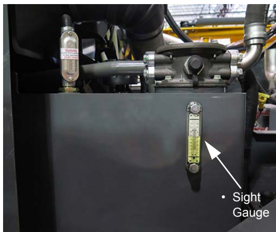
Hydraulic Oil Reservoir (Located on left-hand side of machine - open hood to access) -Typical View
