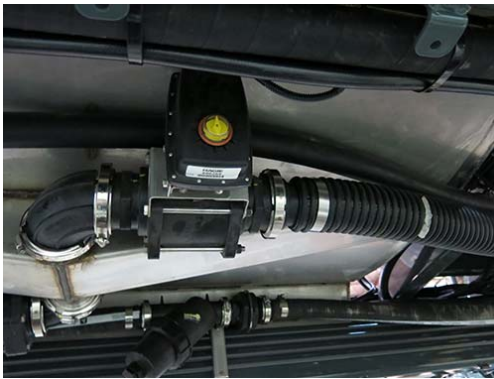
Solution Tank Valve -Typical View
