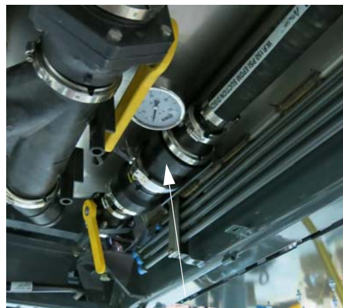
Flow Meter -Typical View
