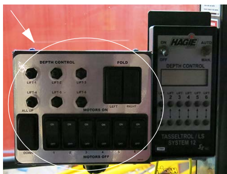
Detasseling Control Panel -Typical View
