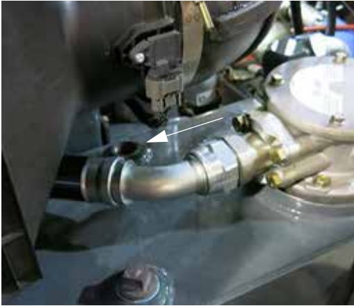
Breather Cap Removed -Typical View
