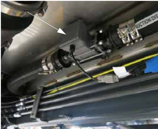
Flow Meter (Located beneath the right-hand side of machine) -Typical View
