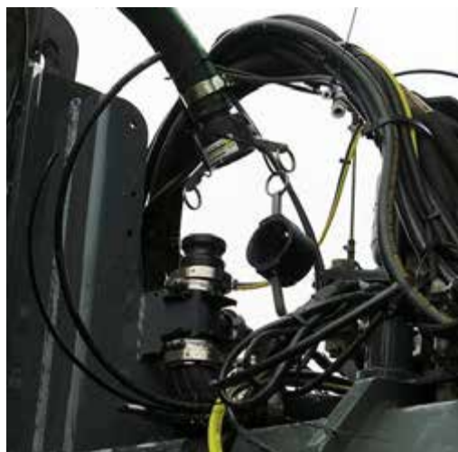
Solution Connection (Located on the front right-hand side of machine) -Typical View
