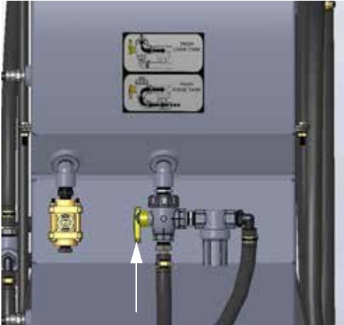
Inlet Selector Valve - 60 Gallon/227 L Tanks (Located on the outer side of Tanks 1 and 3) -Typical View * 3-Injection Pump Configuration
