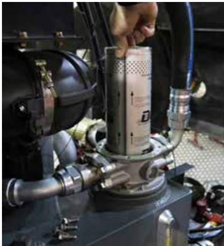
Return Filter (Located inside filter housing) -Typical View
