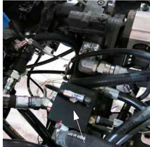
Solution Pump Control Manifold (Located near center of machine) -Typical View
