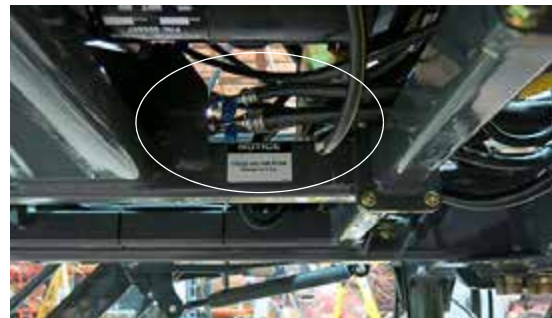
A/C Charge Ports (Located beneath mid mainframe) -Typical View
