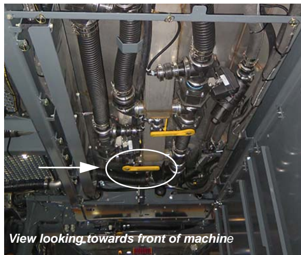
Tank 1 Manual Shutoff Valve (Located beneath center of machine) -Typical View
