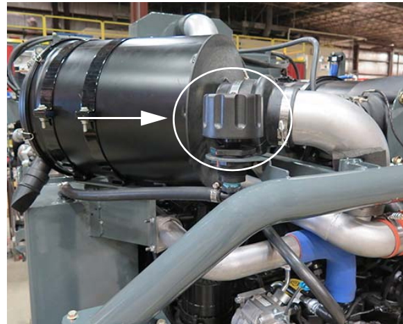
Breather Cap (Located on rear left-hand side of machine behind air intake filter) -Typical View
