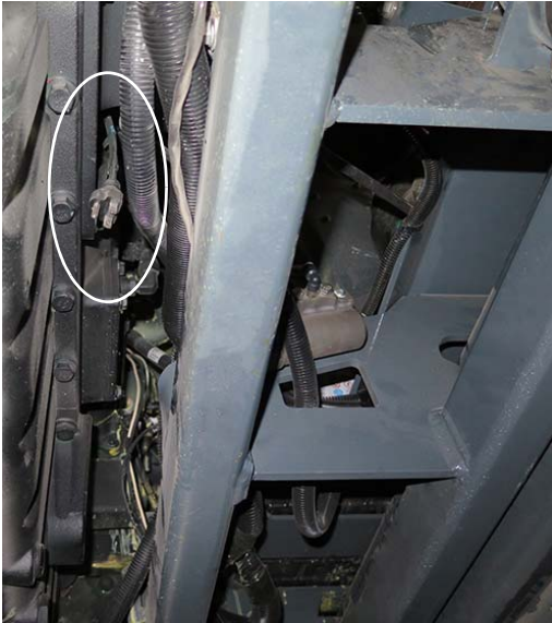
Engine Block Heater Power Cord (Located beneath machine along the right-hand side of engine) -Typical View
