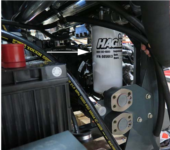
Case Drain Filter 1 (Located on right-hand side of machine near batteries) -Typical View
