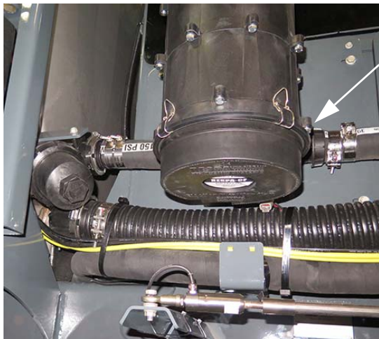
Flow Meter - Secondary (Located near the front right-hand side of machine) -Typical View
