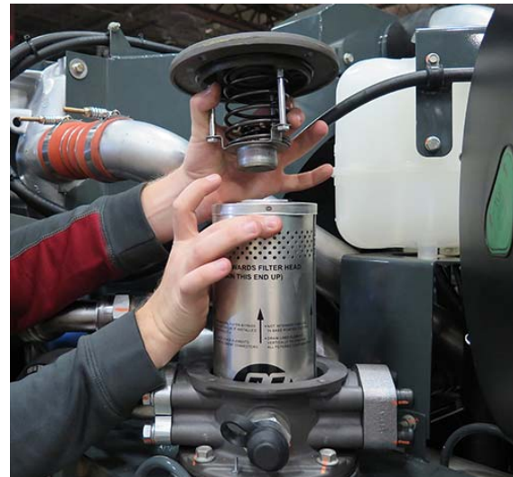
Return Filter (Located inside filter housing on top of hydraulic oil reservoir) -Typical View
