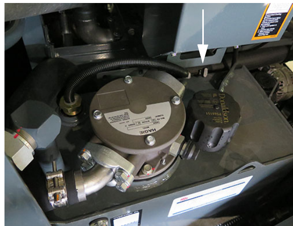
Level/Temp Sensor (Located on top of hydraulic oil reservoir) -Typical View
