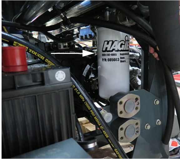
Case Drain Filter 1 (Located on right-hand side of machine near batteries) -Typical View
