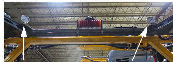
• Secondary Pressure Gauge • Primary Pressure Gauge
