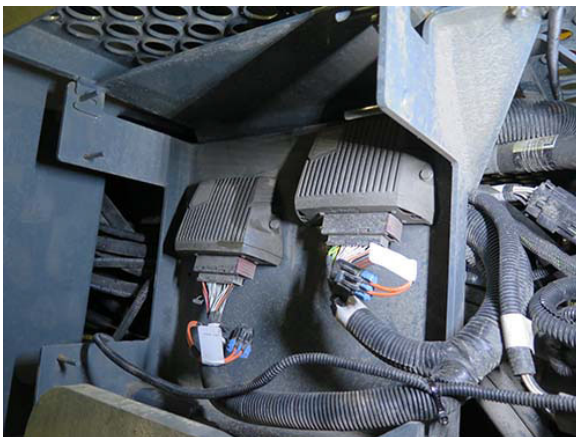
Rear Sensor Power Fuses (Located beneath machine near the rear right-hand tire) -Typical View
