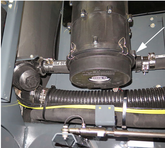
Flow Meter - Secondary (Located near the front right-hand side of machine) -Typical View
