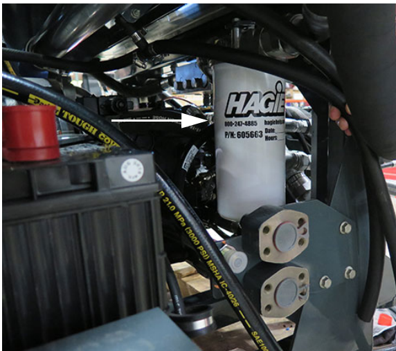
Case Drain Filter 1 (Located on right-hand side of machine near batteries) -Typical View
