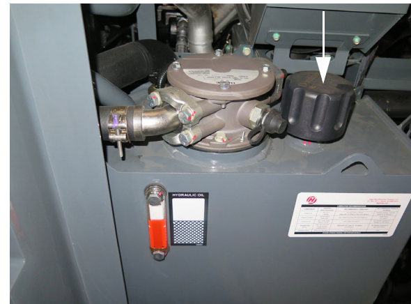
Breather Cap - STS10/STS12 (Located on top of hydraulic oil reservoir) -Typical View
