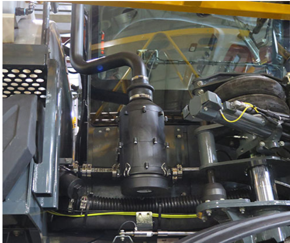
Cab Filtration System (Located on the right-hand side of the exterior cab) -Typical View
