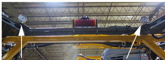
• Secondary Pressure Gauge • Primary Pressure Gauge
