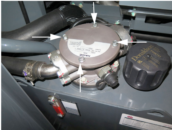
Return Filter Housing (Located on top of hydraulic oil reservoir) -Typical View
